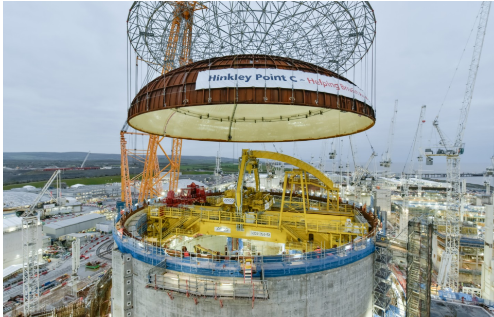
Cap being lifted on to Hinkley Point C number one reactor December 2023
